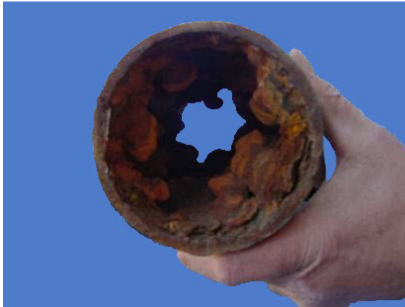
Figure 1: Highly Scaled Pipe from the Plant
